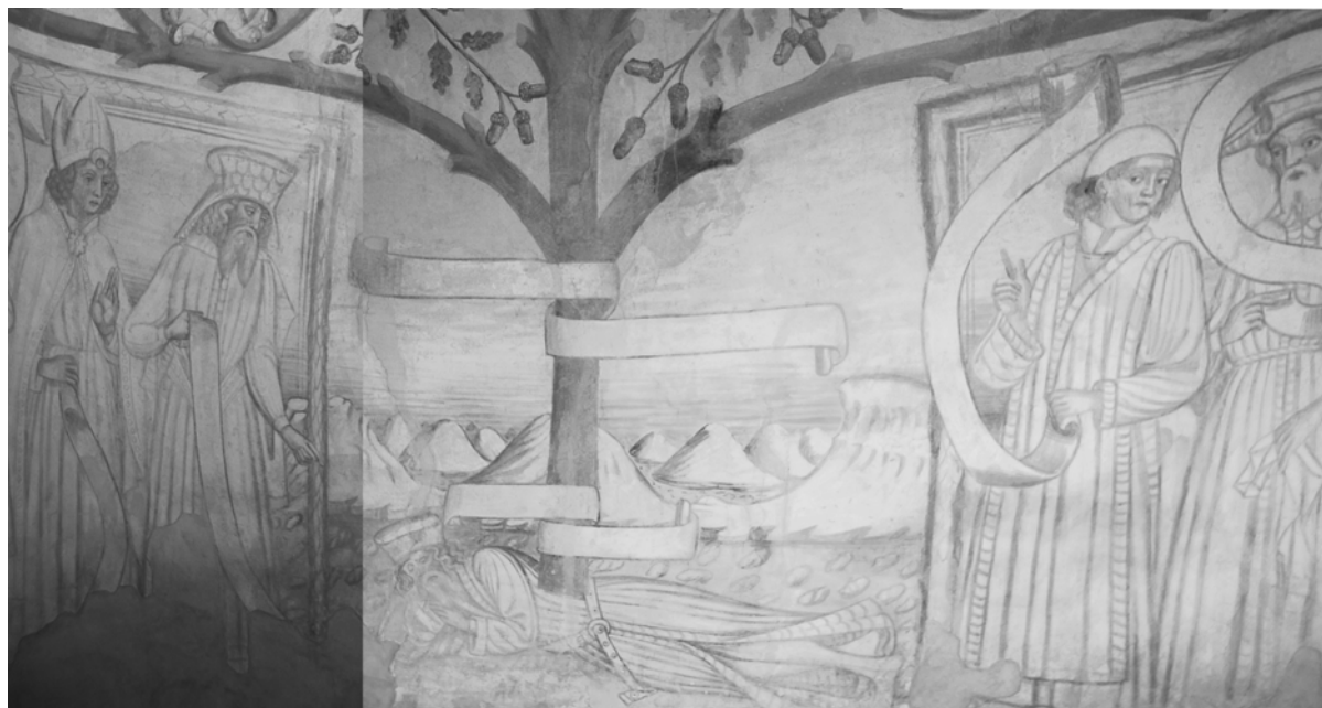
Figure 6. Scaled image mosaic of an orthographic view of the lower central part of the apse
