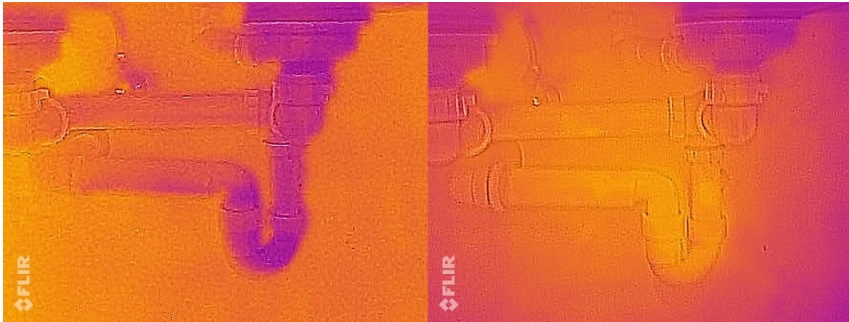
Figure 3.8: Sink trap blocked(left) and fixed (right).
