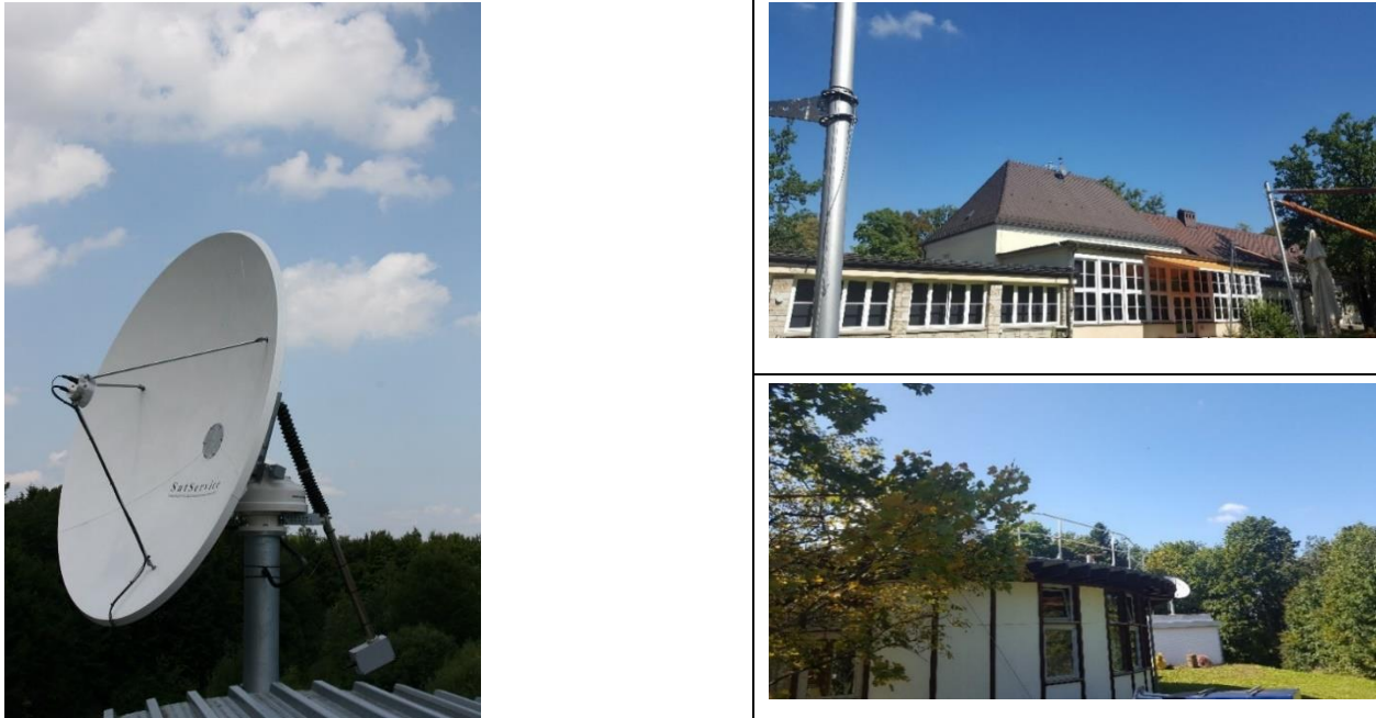
Figure 8: Antenna installations at UniBwM: Dish antenna and geodetic antennas on rooftops.
