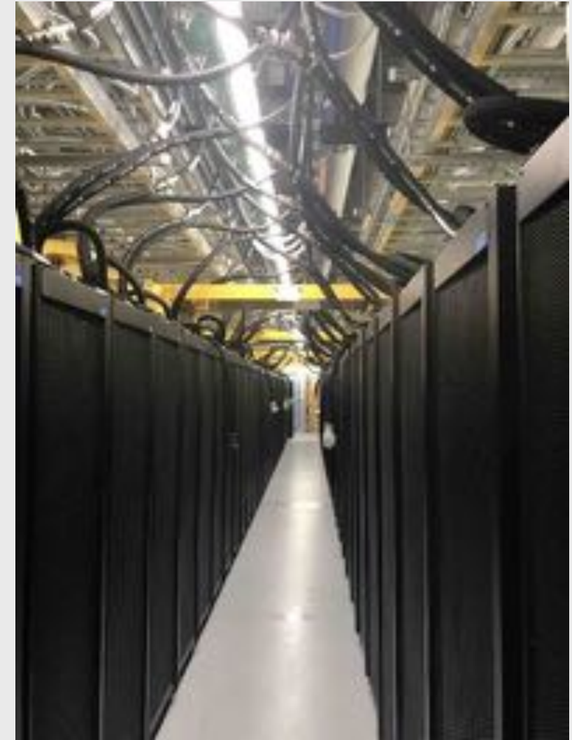
Overhead cooling distribution
